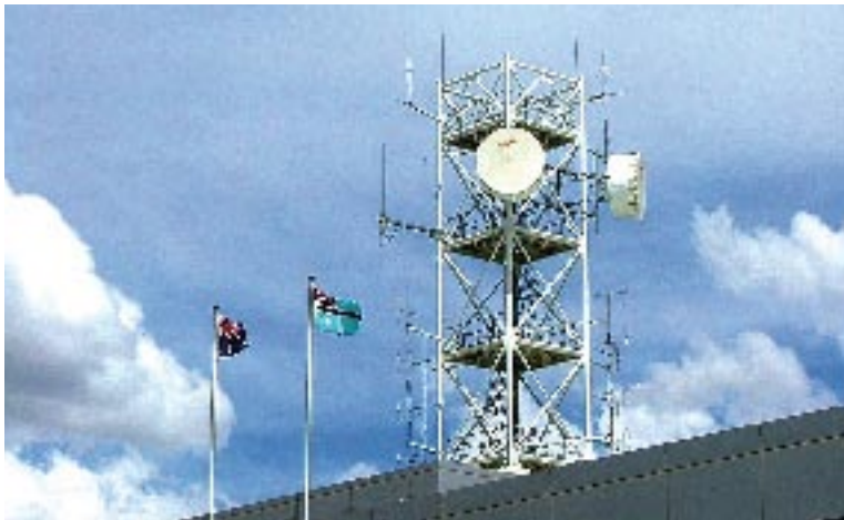
This receiver and antenna system is installed at a field in Germany.
